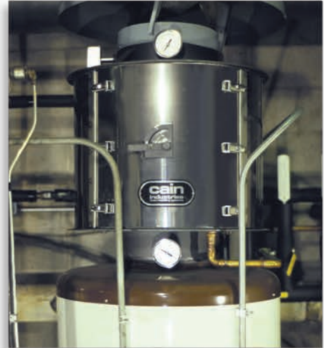
Condominium Complex, Milwaukee, Wisconsin EM Series economizer, on top a domestic hot-water heater, preheating municipal water.
